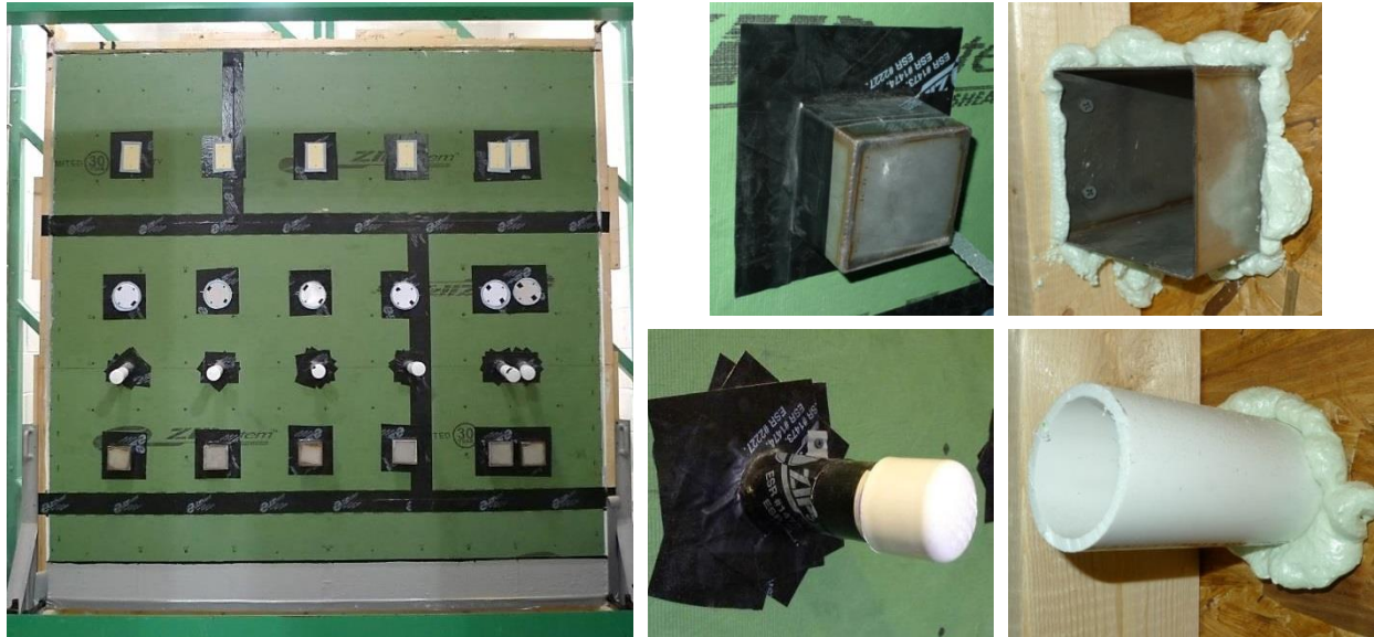
Figure 24. Test wall with OSB with an integrated water-resistive overlay as the air barrier material. Note: We temporarily installed cover plates over the electrical boxes, as shown in the picture above, to evaluate how well we sealed the perimeter of the boxes and the wire holes. We removed the plates before conducting the ASTM E2357 test.
