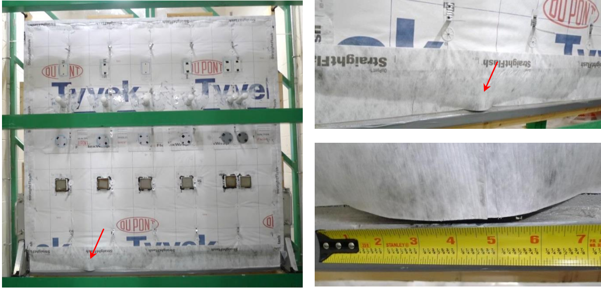
Figure 18. Flashing tape detached from the left side of the CMU during the ASTM E2357 test. Note: We installed cover plates over the electrical boxes, as shown in the picture above, because the flashing tape we used to seal the boxes to the membrane either detached or tore during the ASTM E2357 exfiltration loads. The plates allowed us to conduct the test.
