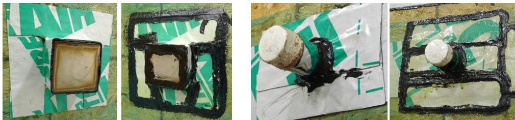
Figure 29. Sealing of steel ducts and PVC pipes was evaluated by measuring air leakage before and after mastic was applied to the perimeter of the membrane.
