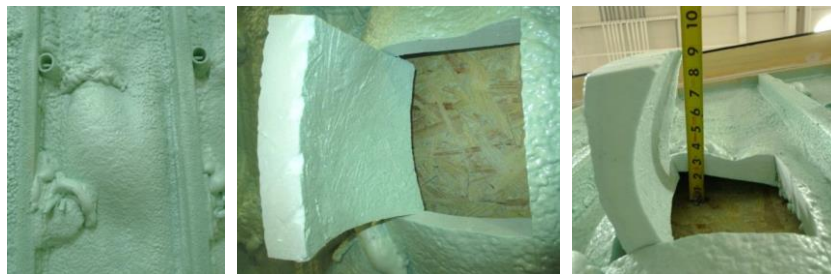
Figure 35. Blister due to loss of adhesion of the sprayed
