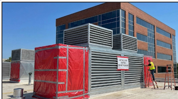
Photo 1: Building Envelope Test: Sealing off the HVAC to test Building Enclosure Material Installation
